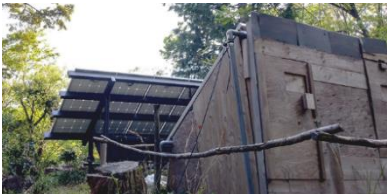
Solar battery panels powering the on-site equipment
