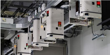
Transport equipment inside the clean room
